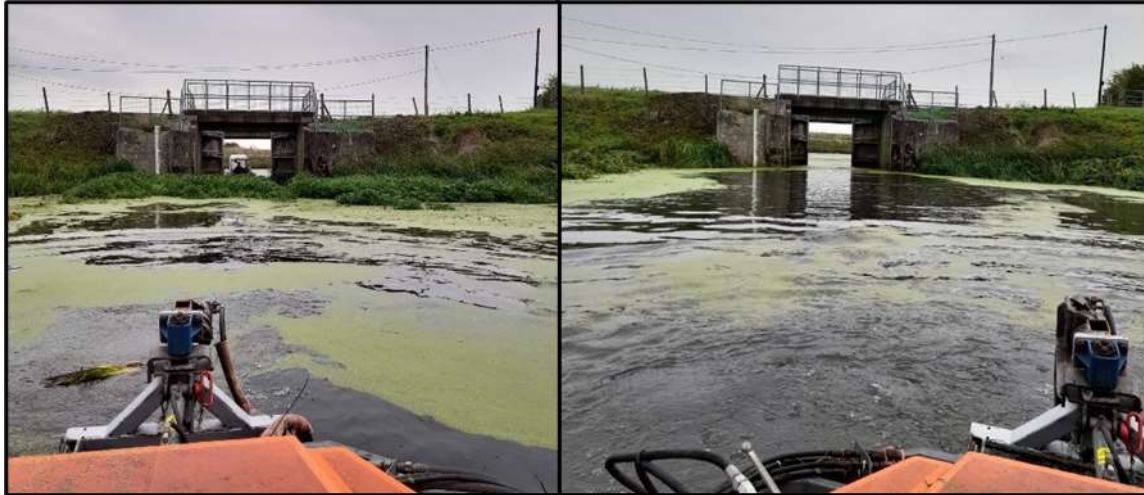
Photos 1/2: Billingham Skirth pointing doors at Billingham Skirth outfall into the River Witham near Tattershall Bridge. Photo (left) show before weed clearance and (right) completed works.
